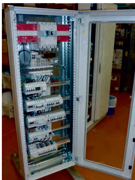
Example: operating test on doors, faceplates, interlocks, etc.
