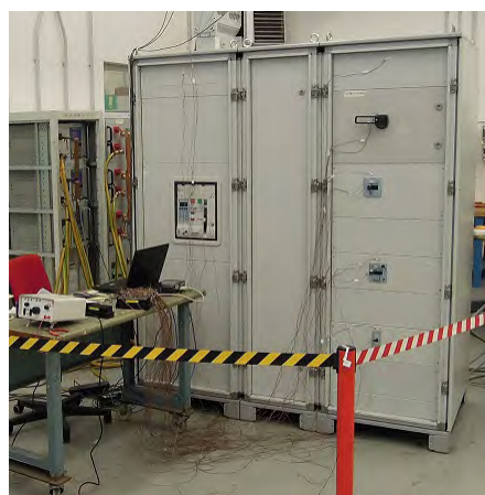
Measurement of the temperature rise limits in an XL 3 enclosure.
