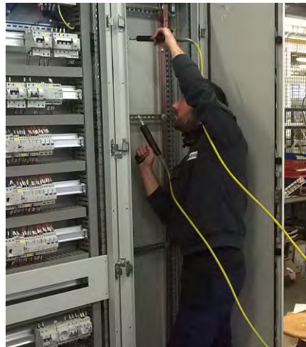
Example: dielectric test at power frequency.
