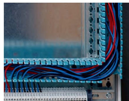
Several circuits in the same trunking and all wiring in vertical and horizontal trunking: column 1 installation
