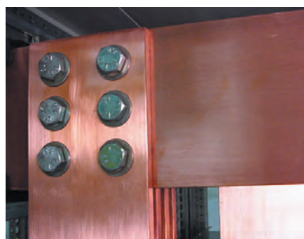
Connection on 120 x 10 bars (4000 A)
