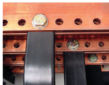
Direct clamping of 5 mm thick flexible bars between two rigid bars with the same spacing
