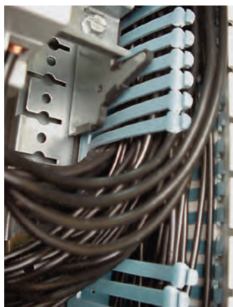
Horizontal circulation “in the open air”, only the vertical conductors are grouped in trunking as here. If the packing ratio of the vertical trunking is high: column 1 installation
